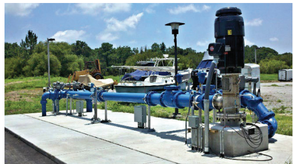
INTERA brings expertise and experience to all phases of groundwater recharge (e.g., ASR, MAR) projects, from conceptual analysis and feasibility studies to wellfield installation, pilot testing, and full-scale operation.
